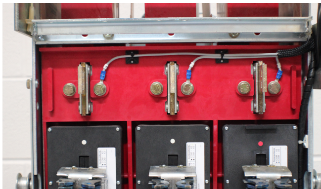
Line-side voltage connections on DS Breaker (Fingers Removed)
